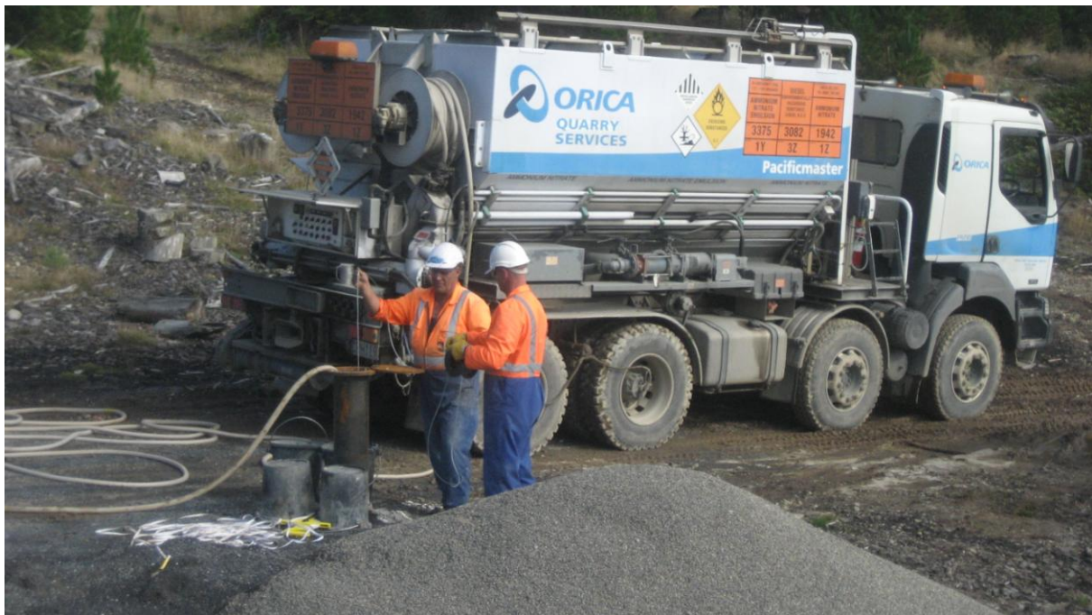
Figure 2.14 Loading of shot hole 11. The MMU truck used to transport explosive emulsion.
