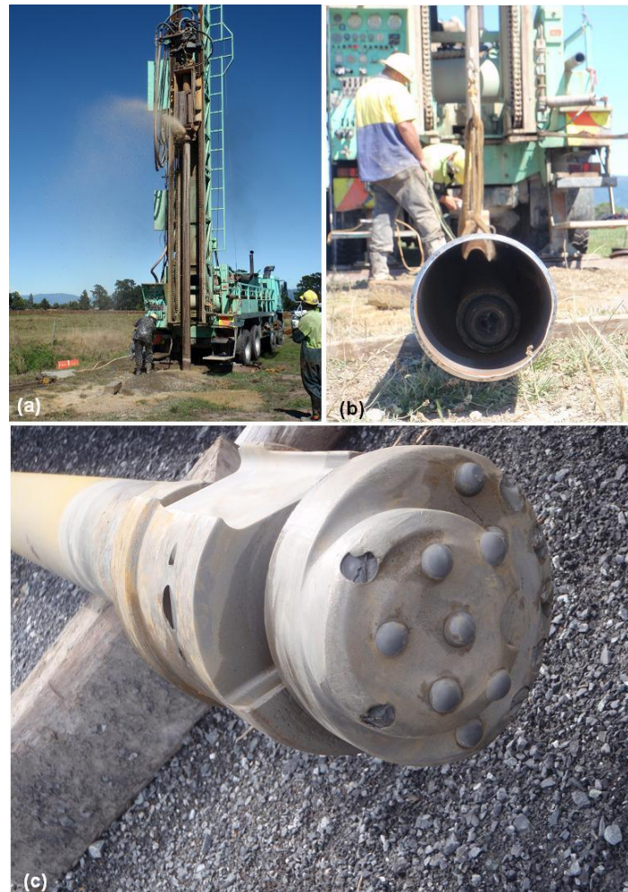
Figure 2.1 Photo (a) shows the drill rig using its top drive casing hammer drilling system; (b) shows the 8in steel casing with a drill bit extension inside; (c) shows the Ecentrix Odex drill bit.
