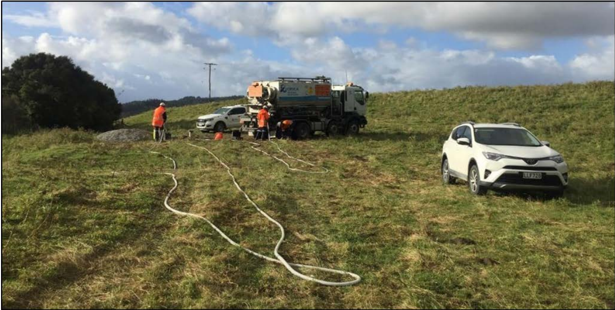
Figure A5.5 Site 1: second blast hole to be loaded. Hose is in the process of being unblocked into a bucket.
