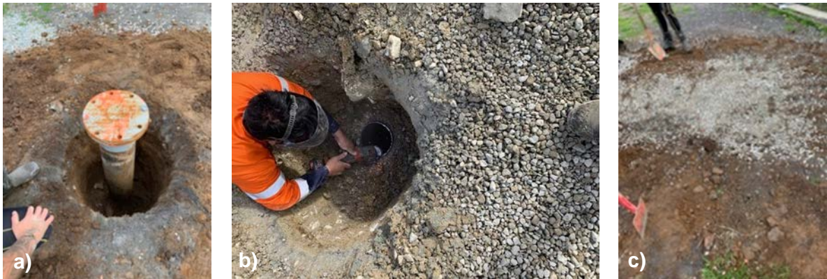
Figure 3.7 Borehole remediation. a) Casing dug out at Site 4. b) Grinder being used to cut casing at Site 3. c) Site 4 after remediation.
