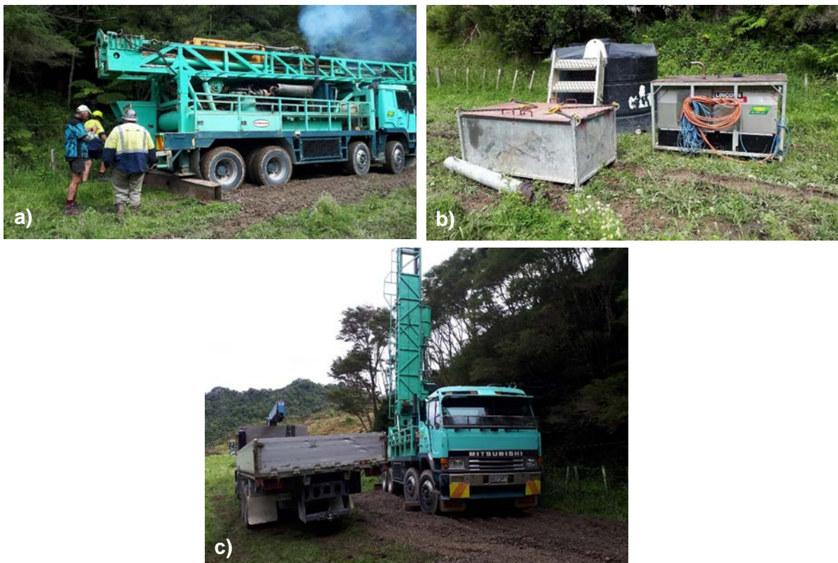
Figure 3.4 Photos of drill rig and equipment setting up at Site 5. a) Drillers positioning the truck to raise the rig. b) Ancillary drilling equipment, including water tank and generator. c) Drill rig raised and truck with casing.
